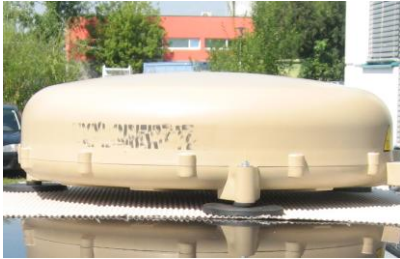
Satellite antenna on roof
