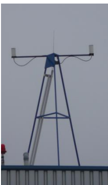
Dual-diversity LOS antennas installed on roof
